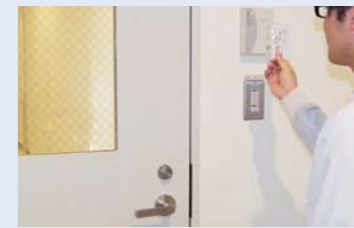
Rigorous security system controls access using ID cards.
